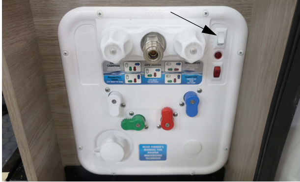
Pump switch -Typical View
