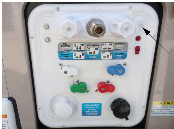
Water pump switch location on Water Center Panel *Model 59K shown -Typical View
