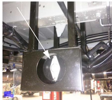
Waste Pump (Located beneath motorhome)
