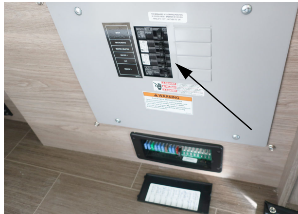
120-Volt Circuit Breakers -Typical View
